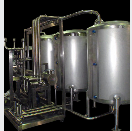
3 tank CIP Set
